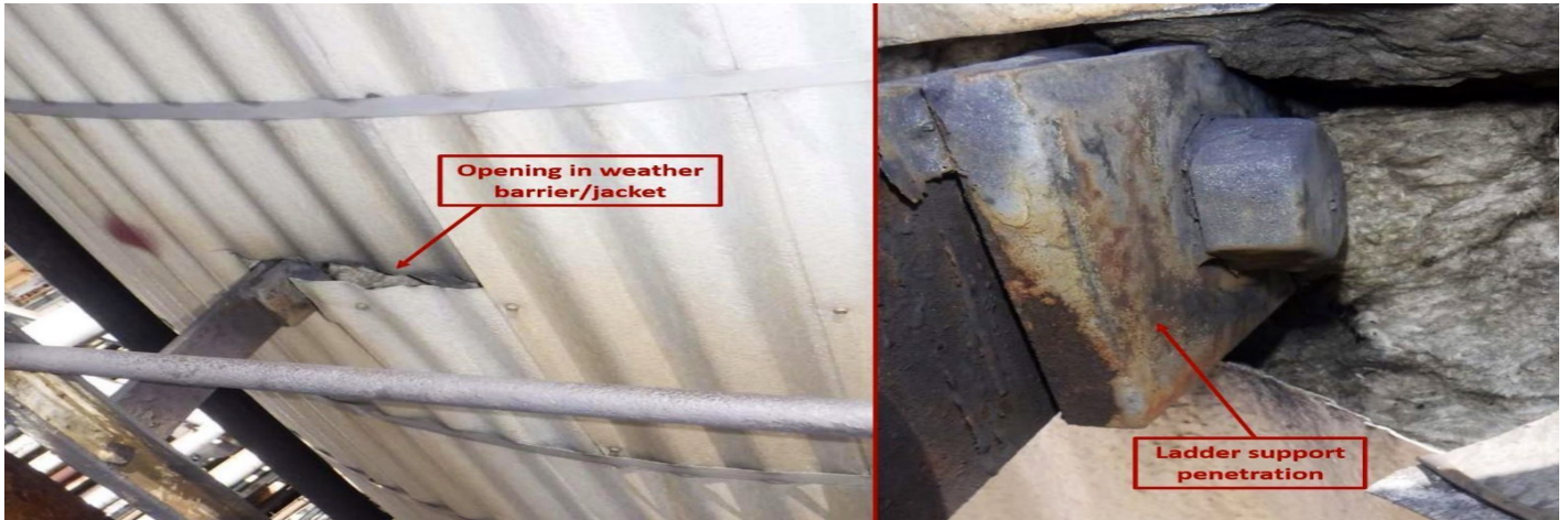
Figure 15. Examples of Unsealed Weather Barrier/Jacketing (Left) and Close-Up of Ladder Support Penetration (Right) on a Vertical Pressure Vessel.
