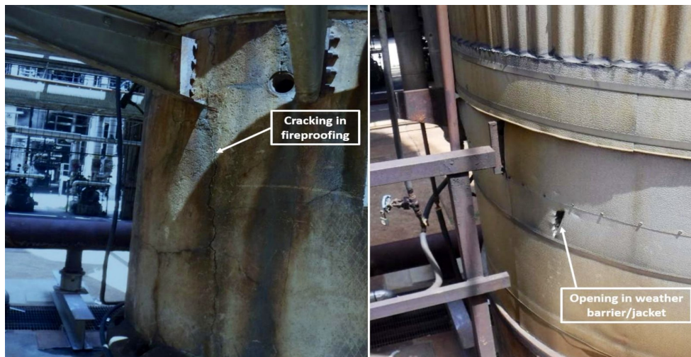
Figure 14. Examples of Degrading Fireproofing on a Support Skirt (Left) and Damaged Weather Barrier/Jacketing on a Vertical Pressure Vessel (Right).
