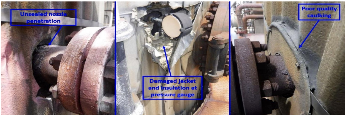
Figure 16. Additional Examples of Improper Insulation System Design at Nozzle and Instrumentation Penetrations.
