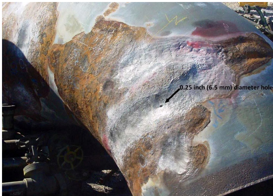
Figure 8. Example of a Small Diameter Hole (Pinhole Leak) in a Carbon Steel Pipe Due to CUI [4].
