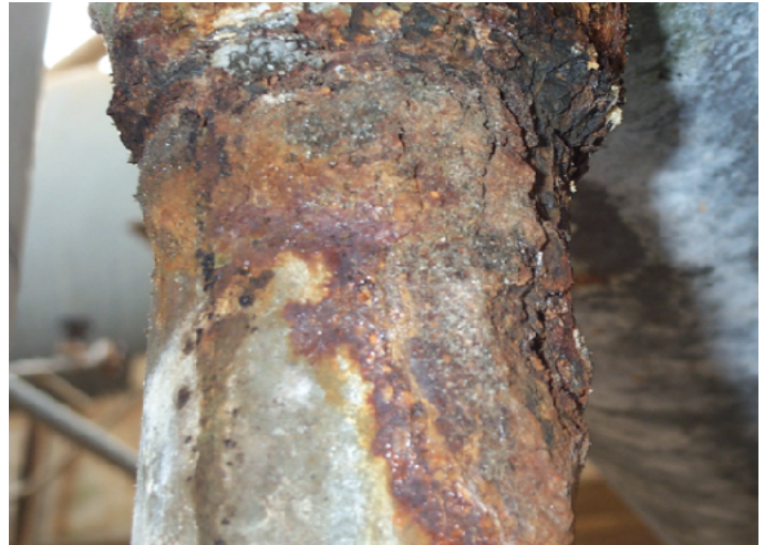
Figure 3. Close-up of CUI (Localized Corrosion) of a Piping Tee after Insulation Removal [3].
