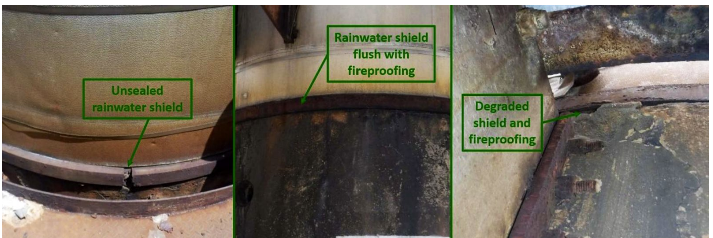
Figure 17. Examples of Poor Design Details, Installation, and Maintenance Practices Near Rainwater Shield at Support Skirt Fireproofing-to-Shell Insulation Junction.
