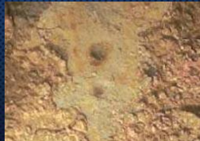
Pitting corrosion of SS
