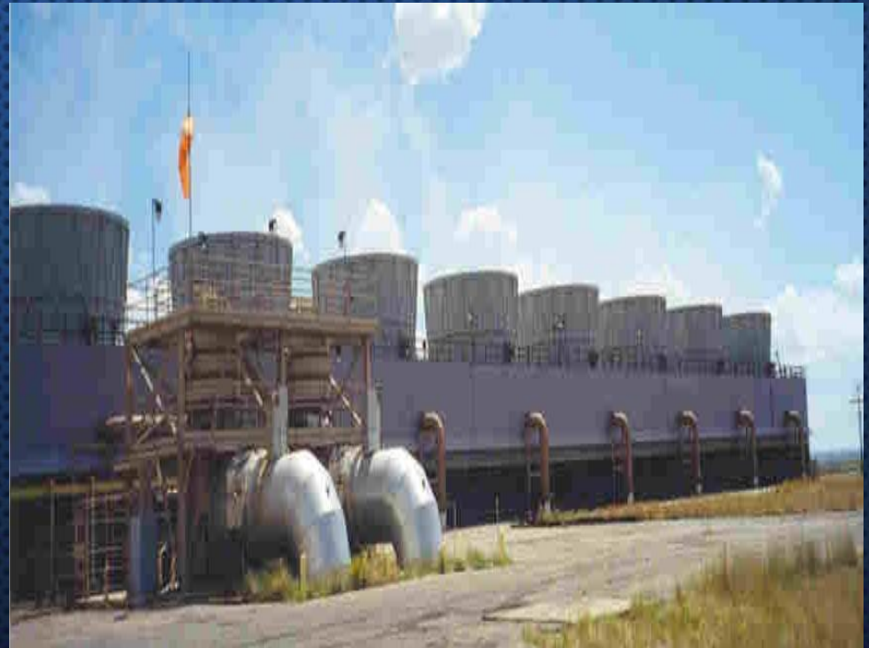
A Cooling Tower Unit
