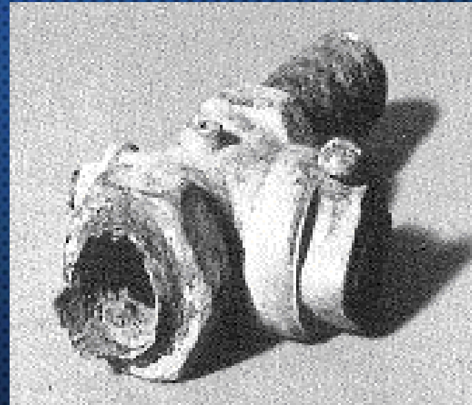
Galvanic corrosion of steel pipe at brass fitting in humid marine atmosphere
